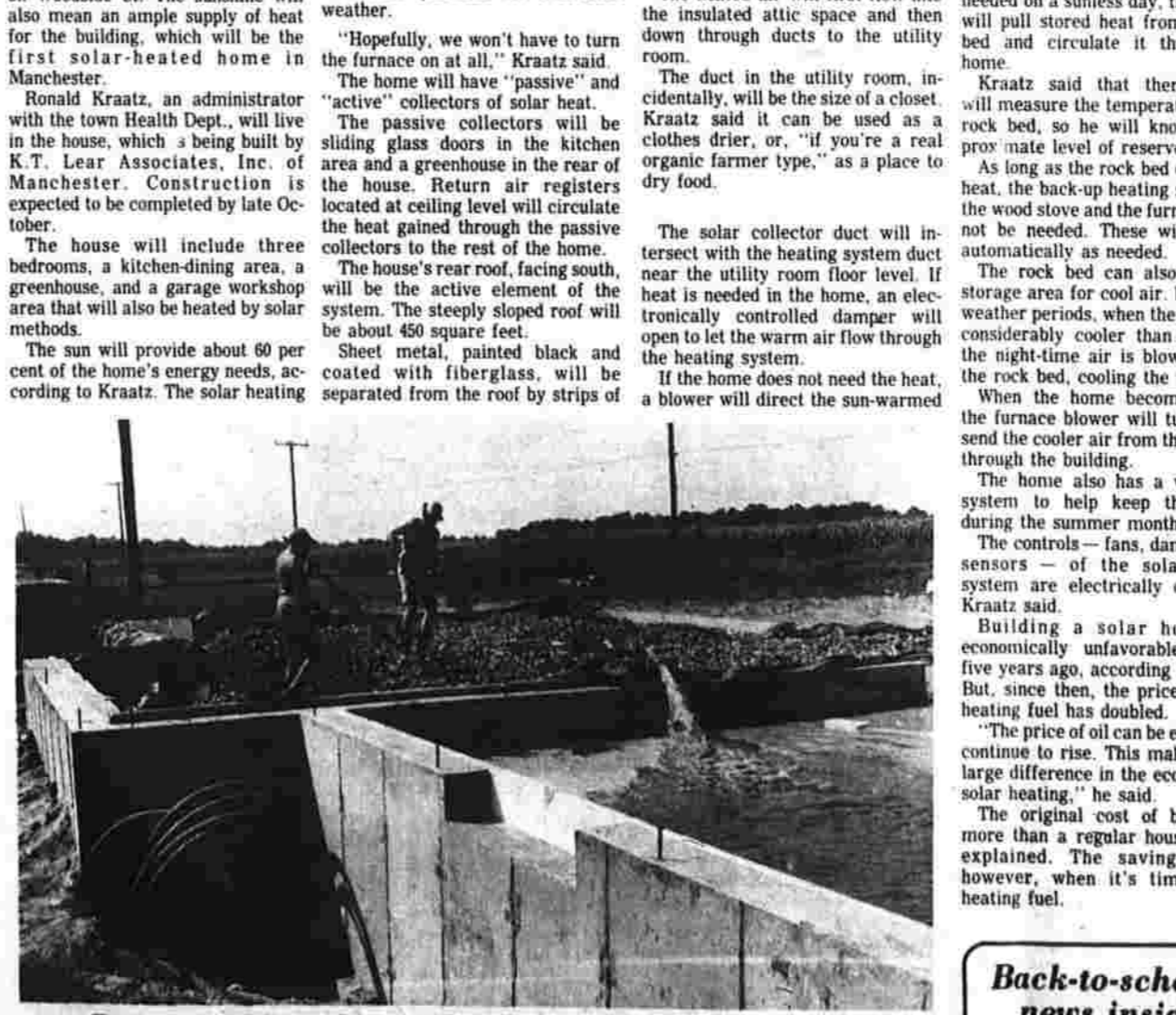
Preparing foundation for solar heated home Bill Wenzel (left) and Al Eggen (right) of K.T. Lear Associates work on washing and leveling stones in the foundation of a solar-heated home being built on Woodside St. The rock bed, which contains 50 tons of stone, will act as the storage area for excess solar heat taken in by the home's collector. (Herald photo by Dunn)
